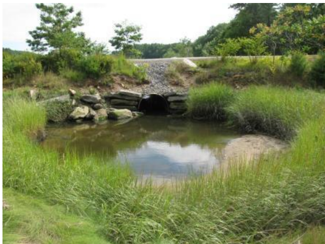
Thomas Bay Salt Marsh Restoration, Adams Road inlet, pre-construction, 8-9-2011. Photo courtesy of Matt Craig of the Casco Bay Estuary Partnership.
